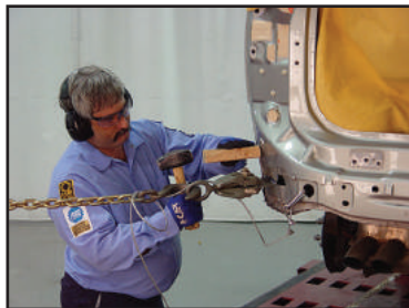
Figure 5 - A pulling plate welded to a part made from UHSS alloyed with boron is used to remove indirect damage.
