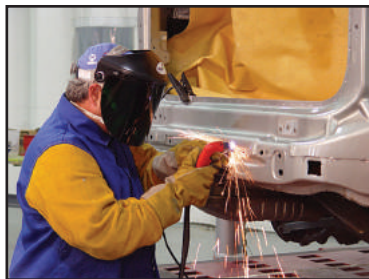
Figure 4 - Plasma-arc cutting equipment can be used to cut around the spot weld.
