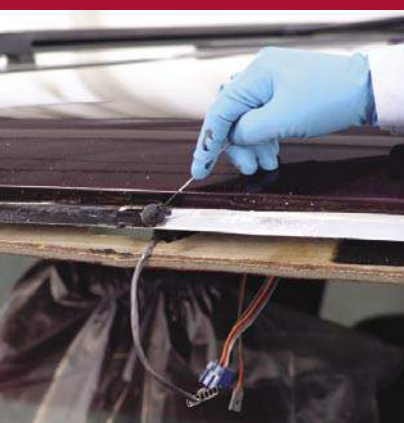
Figure 6 - Pinchweld primer, specific to the urethane being applied, must be applied over the corrosion-resistant primer before applying the urethane.
