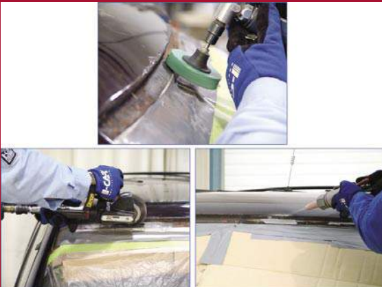
Figure 4 - Common methods of corrosion removal include using a plastic-coated abrasive wheel, wire wheel, and a media blaster.
