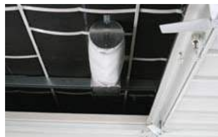
Figure 3 - The intake filter for the Junair QAD system is located in the spraybooth plenum.
