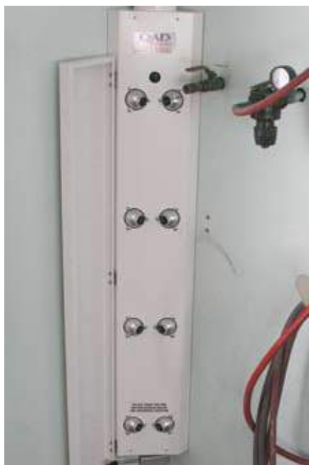
Figure 2 - The Junair tower contains eight nozzles that can be adjusted manually for optimum airflow.
