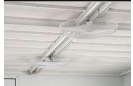
Figure 6 - The ceiling fans are installed down the middle of the spraybooth.
