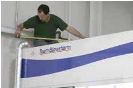
Figure 4 - The ductwork is run outside of the spraybooth to the blower motor located on top of the spraybooth.
